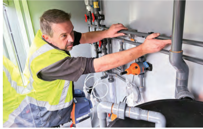
NPDC's Clive Fleming, with the equipment that will introduce fluoride into New Plymouth's water supply the end of this month.
